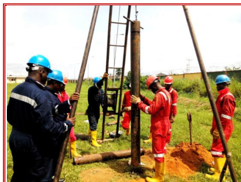
Figure1: Drilling by Percussion Method of one of the Boreholes in Process during the study
